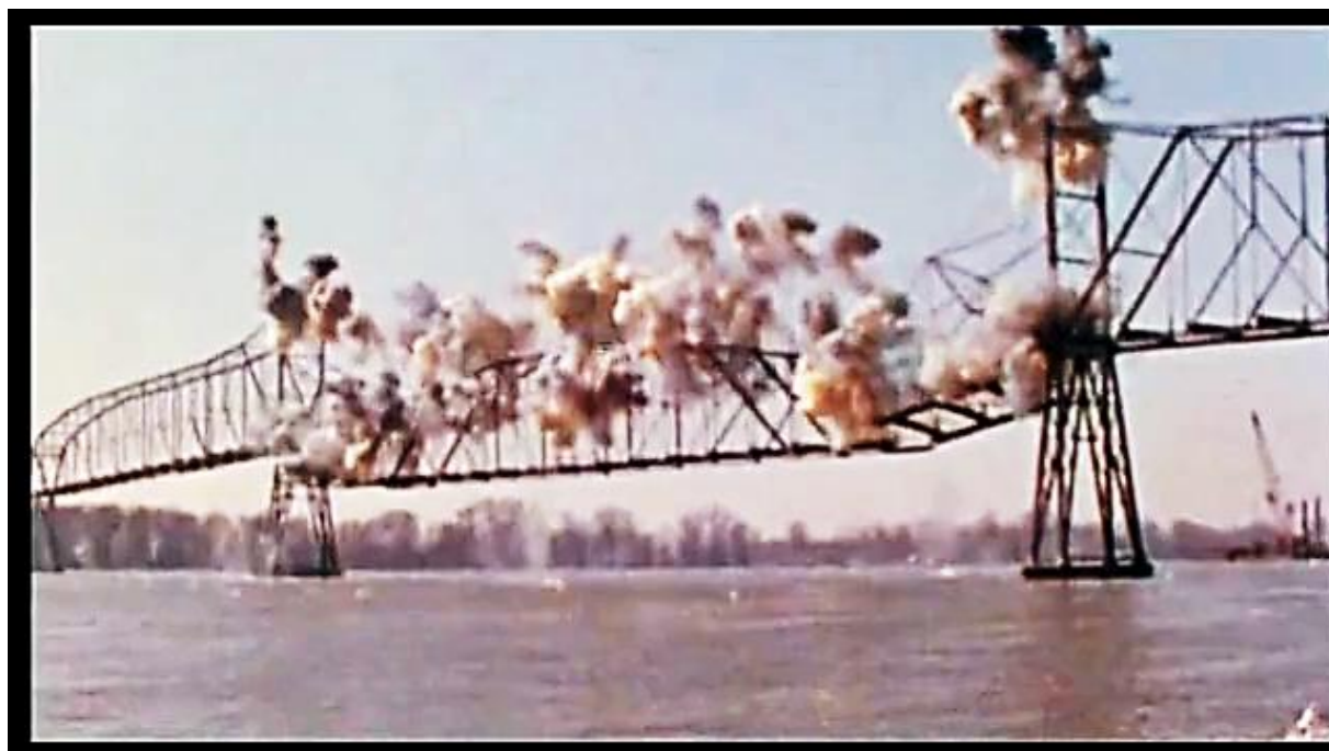
Figure 1. Bridge Demolition , Koyaanisqatsi , dir. Godfrey Reggio, score Phillip Glass, cinematography Ron Fricke, Institute for Regional Education, 1982, 35:32.
